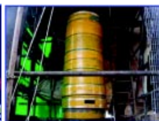
Fig 24 – Repair sleeves cut to suit the axial length plus bridging girth welds.
