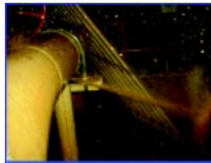
Fig 5 – Ongoing leak on the separator tee.
