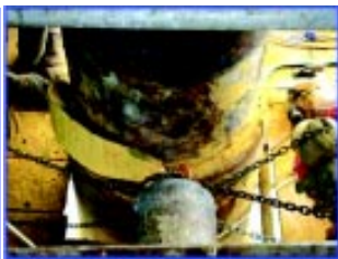
Fig 22 – Corrosion underneath the clamp.
