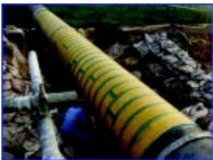
Fig 19 – Completed composite coil installations.
